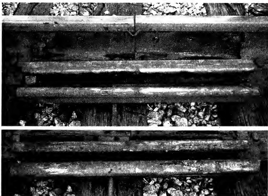
Fig. 7. North Portion Section 2, Conoco Anti-Rust Compound with Plastic H Plugs in Both Ends (Brush coat on rail and bars)
